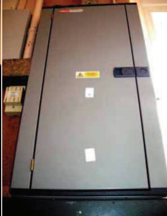
Barrhill Hall 3 phase distribution board
