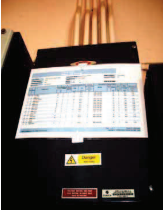
Barrhill School 3 phase distribution board
