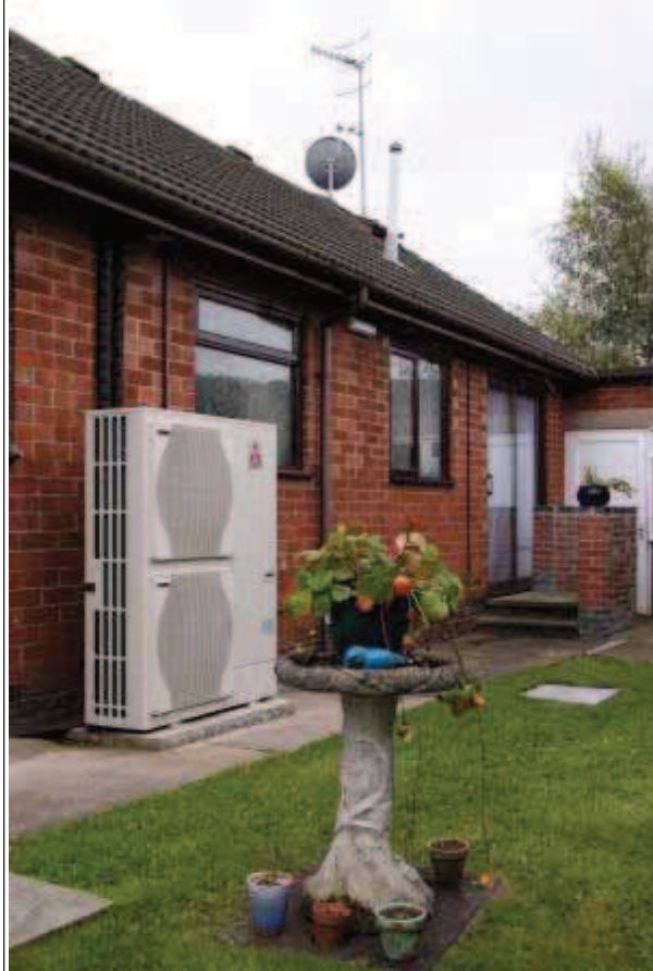
Typical 14kW air source heat pump installation
